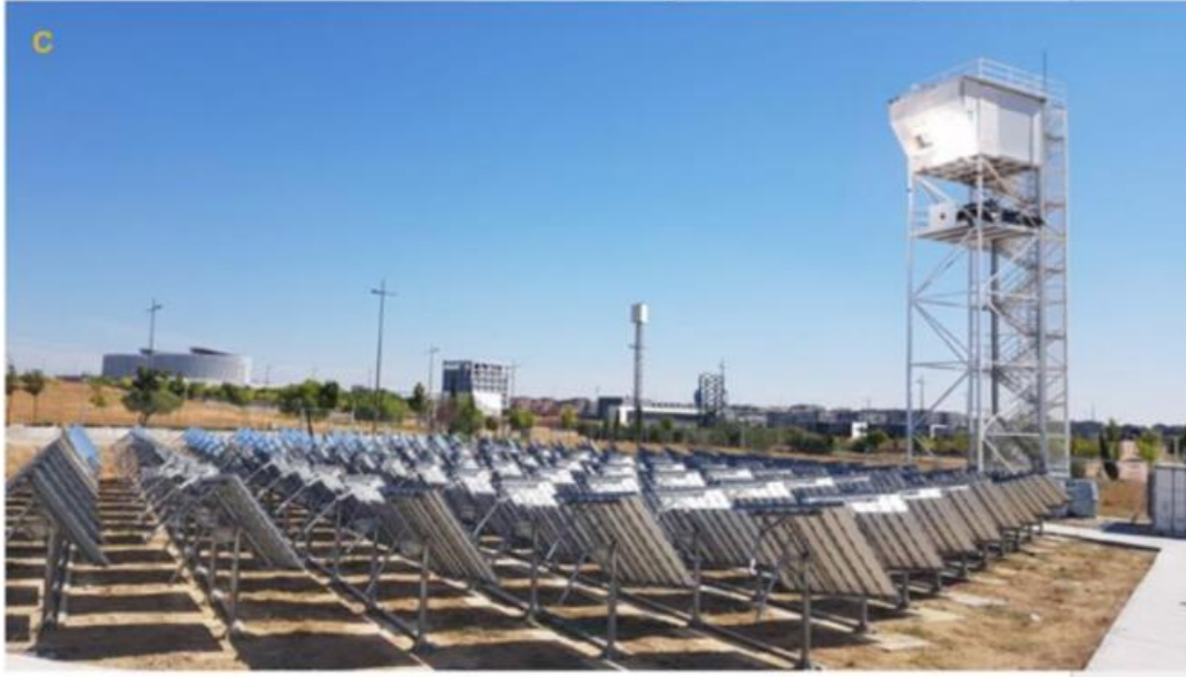
Figure 14: Experimental tower at IMDEA in Madrid
